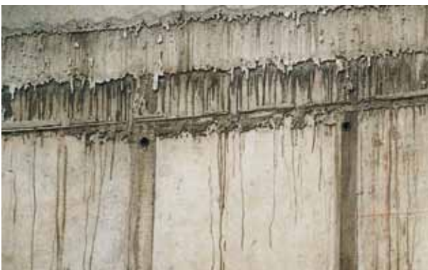
New concrete with laying defects requiring subsequent filling
