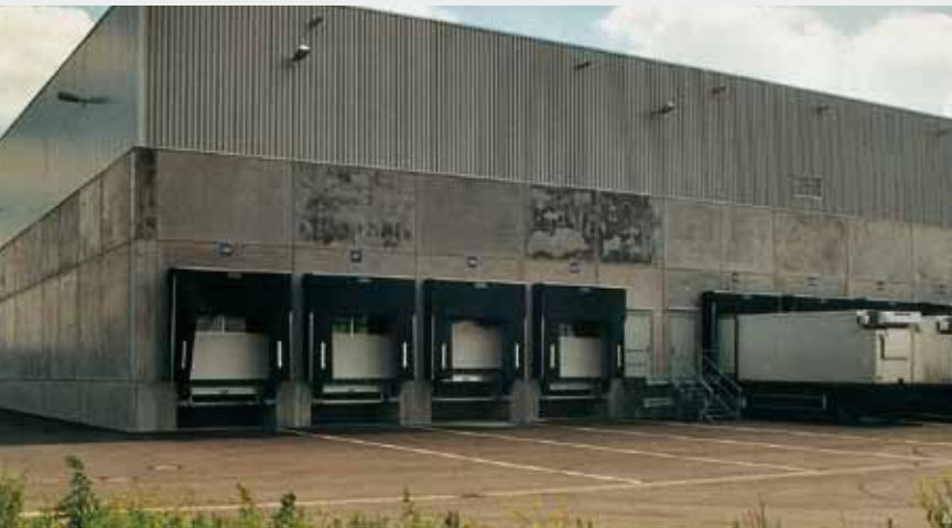
Uneven, unattractive appearance
