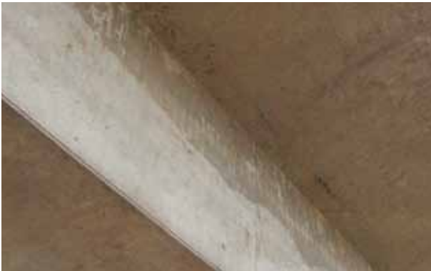
New concrete with slight blemishes
